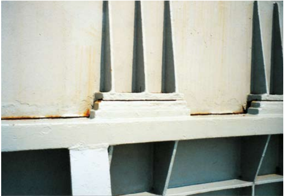
WORN 'STEEL-TO-STEEL' CONTACT POINTS.
